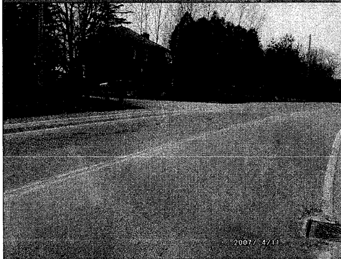
Areas of alligator cracking and patching in southbound lane
