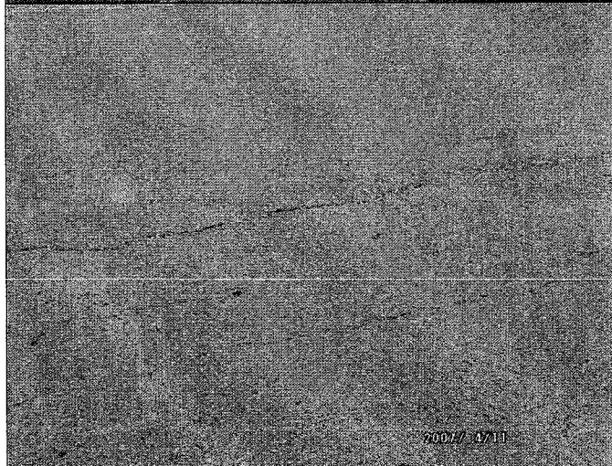
Typical longitudinal cracking.
