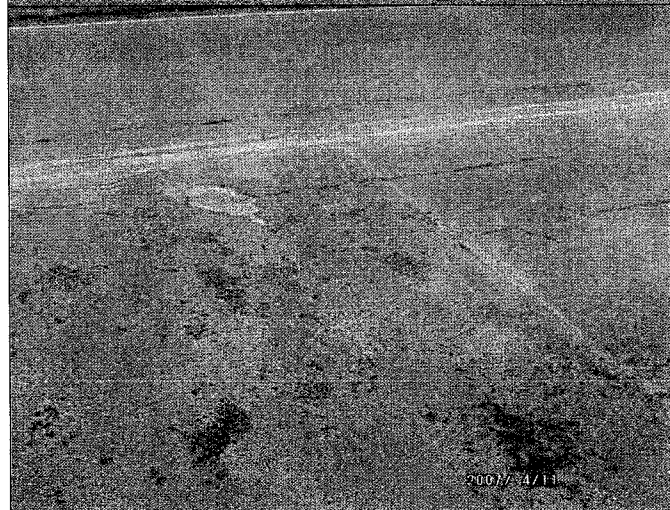
Distress area in northbound lane. Note delamination of overlay in upper right corner of patch.
