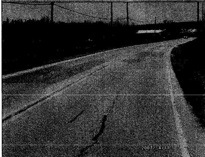
Typical patches and cracking in centre section of project.
