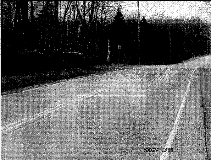
Typical longitudinal and transverse cracking in northern section of project.
