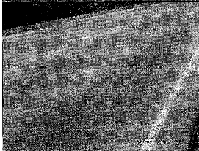
Cracking and rutting in both lanes.
