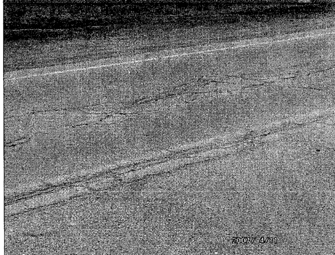
Distresses in southbound lane.
