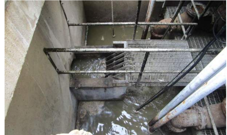
Wet Well, with View of Screen and Pump Discharge Pipes
