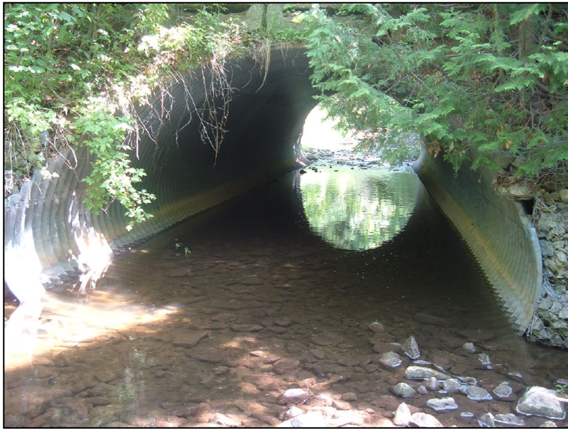
Figure 5.7 Monitoring Station T1 (North Branch of Black Cr. at 6 th Line) Channel Cross- Section
