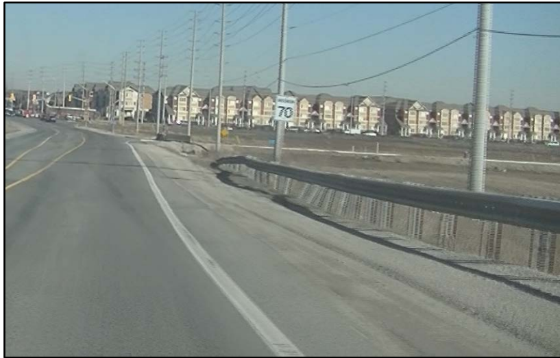
Figure 24: Poor Condition of Guide Rail located north of 407 ETR Northbound On-ramp
