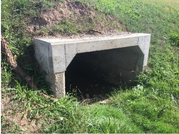
Photo 3: Box culvert on the east (upstream) side of Ninth Line at location 604764E 4818651N
