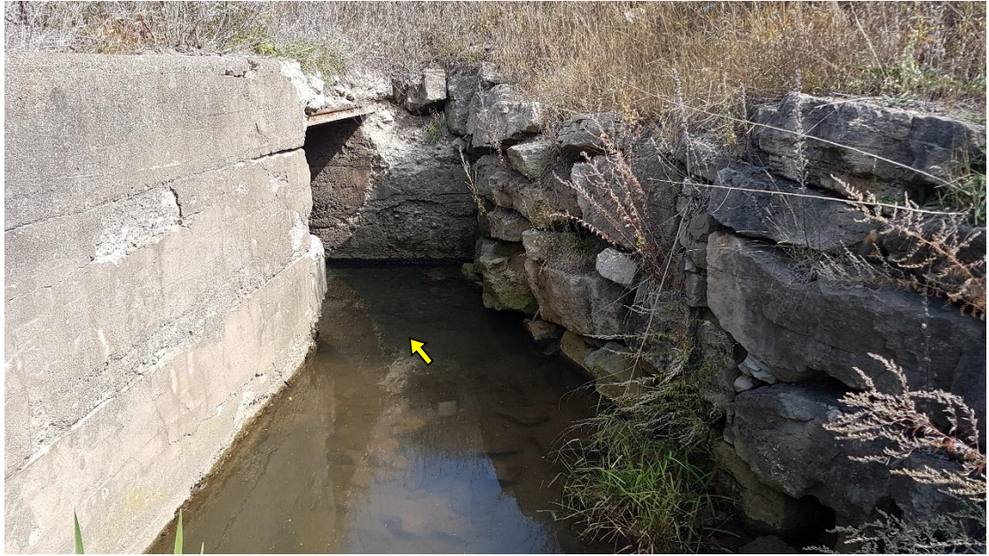
The supporting headwall and concrete retaining walls of the plunge pool were degraded and in poor condition.
