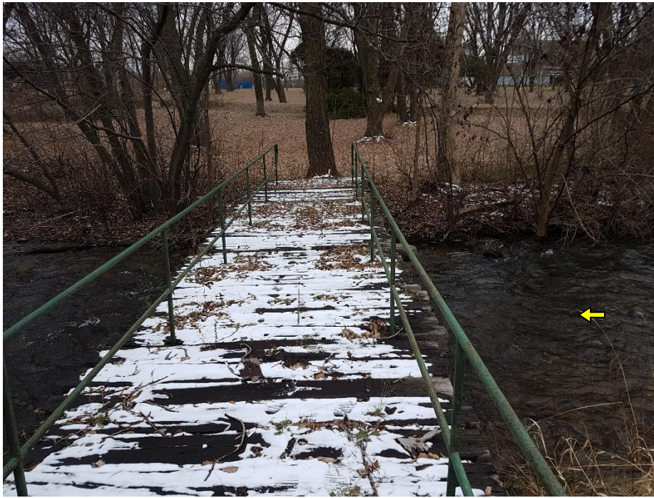
An additional wooden bridge was noted 180 m downstream of the Steeles Avenue crossing. The adjacent channel banks were vegetated and moderately stable.
