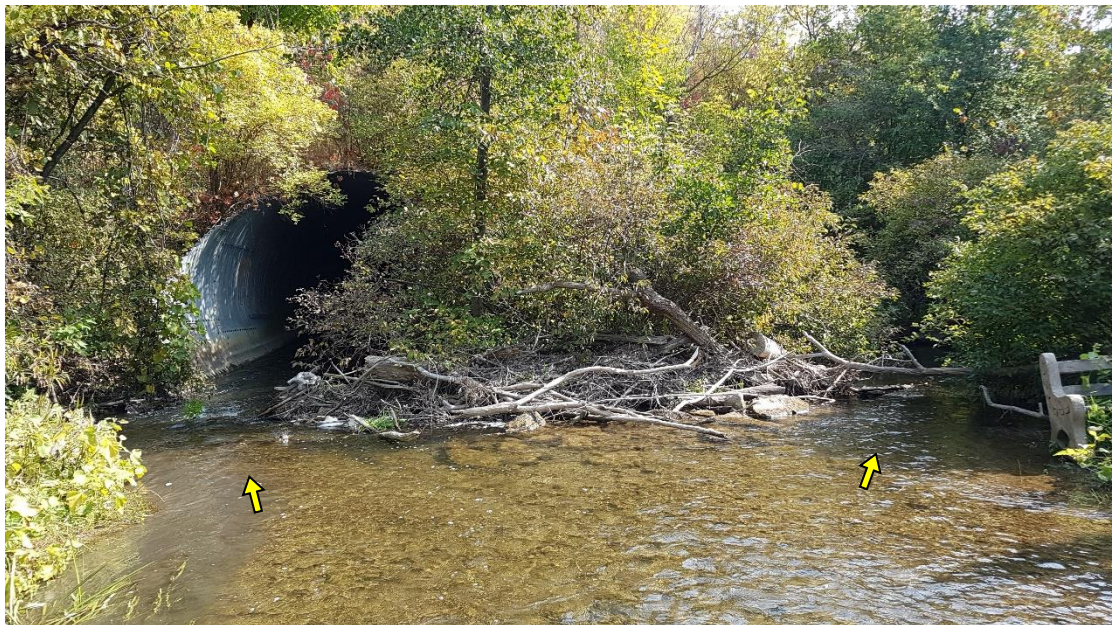
The CNR crossing of Sixteen Mile Creek consisted of two 3 m x 4 m culverts. Woody debris had collected along the bank between the culverts.
