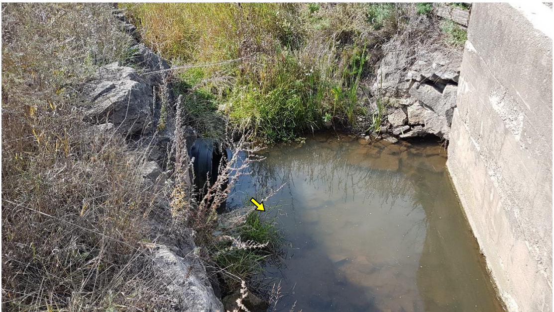
NW-1-E was conveyed beneath Steeles Avenue within a 750 mm diameter corrugated plastic pipe. The channel fed into a stone-lined plunge pool at the base of the road / rail embankment.
