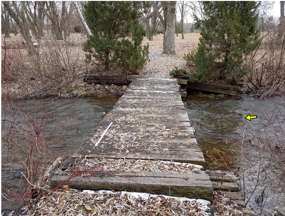
100 m downstream of the crossing, there was a wooden bridge associated with the Milton Banquet and Conference Centre lot. The bridge was partially-rotted, though not displaced.
