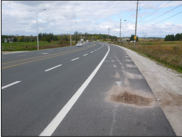
Plate 1: Field conditions within the study corridor, facing northwest. Note disturbance within the ROW, and areas of archaeological potential outside the ROW.
